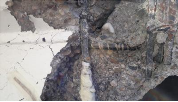
Fig. 8 BFRP failure in B-19
