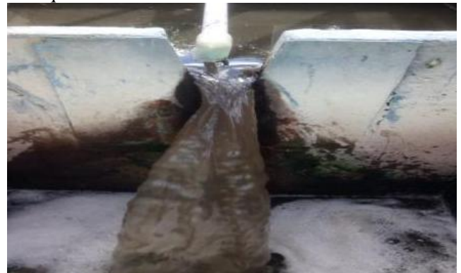
Fig. 18 Application of anionic flocculant in discharge dump to flocculation tanks
