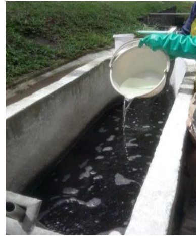
Fig. 16 Application of peroxide in the gutter of the water treatment plant of Industrias Printex S.A.S.
