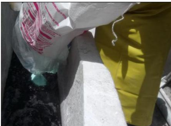
Fig. 15 Application of ferrous sulfate heptahydrate in the gutter of the water treatment plant of Industrias Printex S.A.S.
