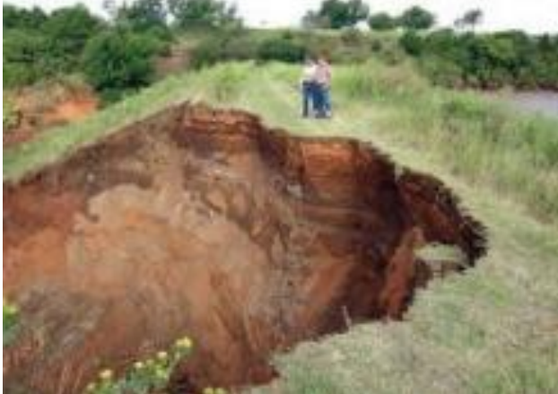
Fig. 2 Dam erosion due to the rainfall
